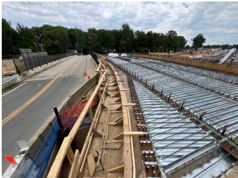
Aluminum deck pans on the right will hold in place the poured concrete. The new bridge is anticipated to open in late July (June 2024).
