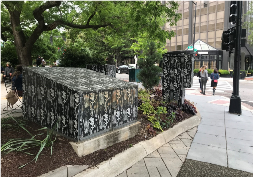
Above: Utility cabinets at Duke Ellington Park, Washington, D.C. Image: Fairfax County Staff.
